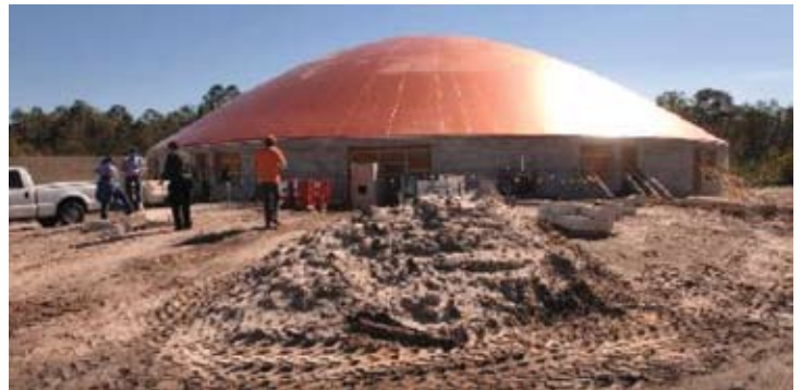
The first of five dome-covered buildings that will make up The Children's Reading Center Charter School in Palatka is beginning to take shape through the efforts of GMC Construction of Gainesville. BRUCE LIPSKY/The Times-Union
